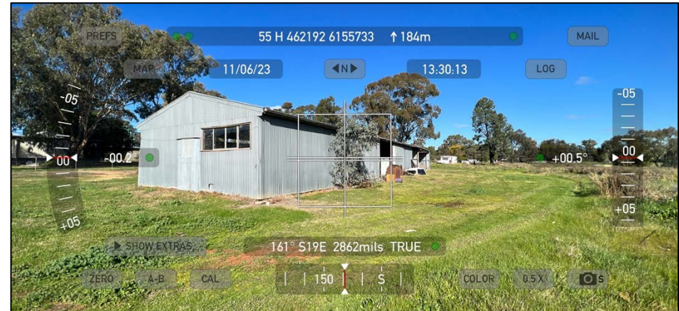
Photo point 11 Looking at the general condition of the existing shed to the west of the existing residence.
