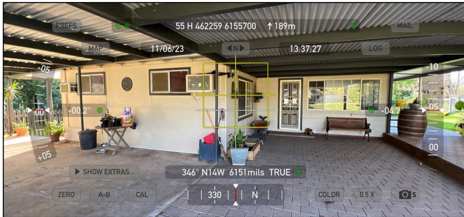
Photo point 5 Showing the general condition of the existing residence south elevation.
